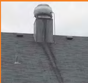
Unattractive Roofs, Parking Lots, & Floors
